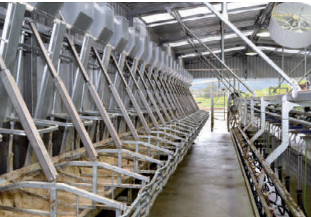
Powering the stall gates with a pneumatic ram eased the demand on the dairy's vacuum pump.
