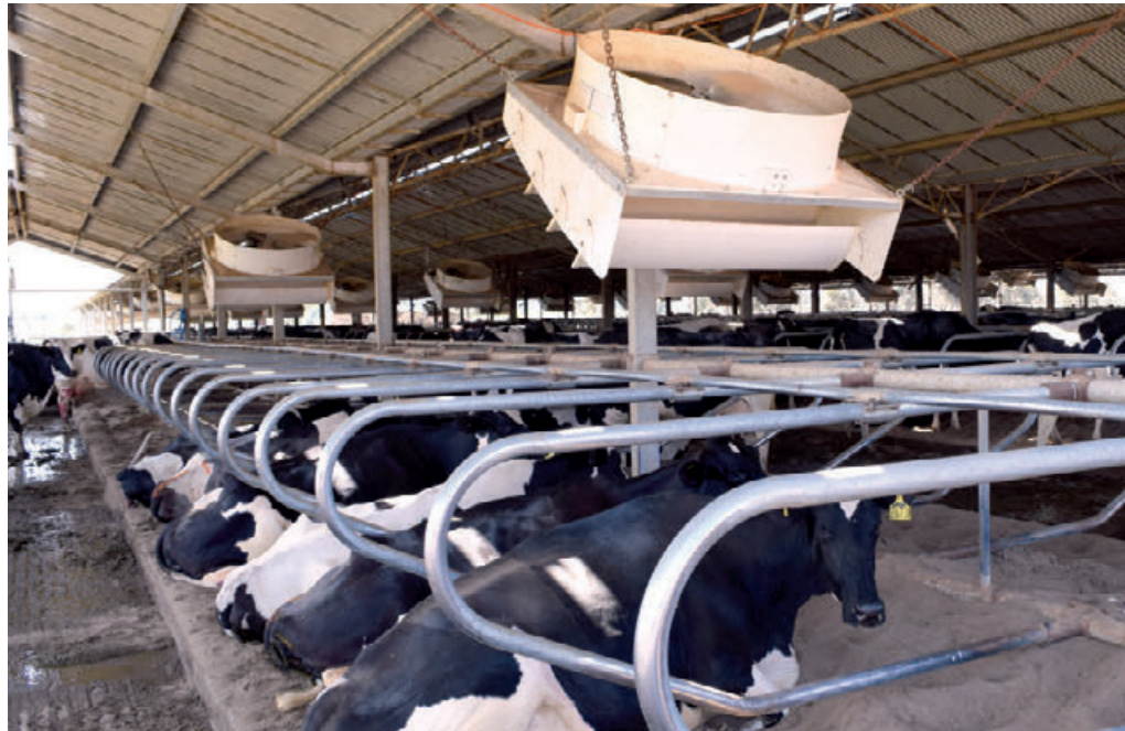
Fans installed at the end of 2017 made a big impact this summer, helping hold Silvermere's average per cow production through January at 41 litres.
