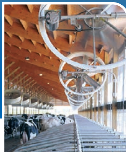
Daviesway distributes VES-Artex Barn Solutions in Australia because the US-based company has unmatched knowledge in cow cooling conversations.
